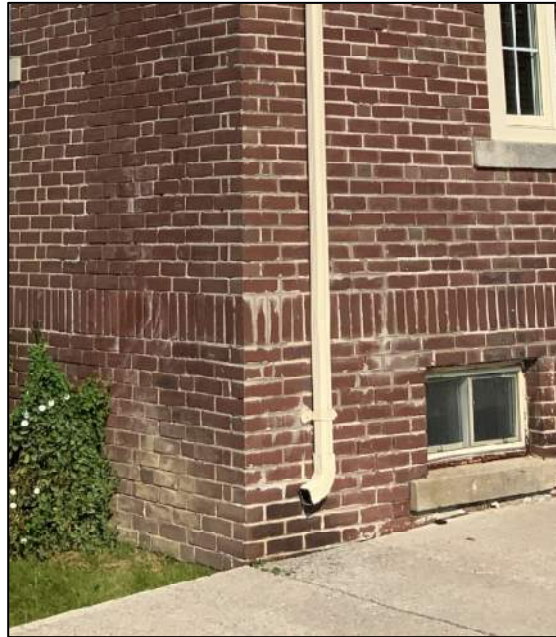
Photograph 4: Poorly executed masonry repairs (typical)
