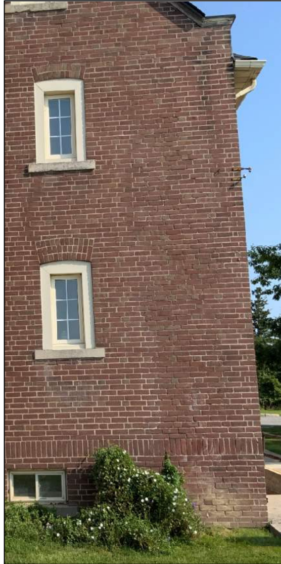
Photograph 3: Mortar deterioration at south elevation, east corner
