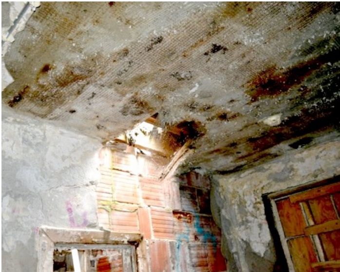
Mold apparent in lath and concrete ceilings.
