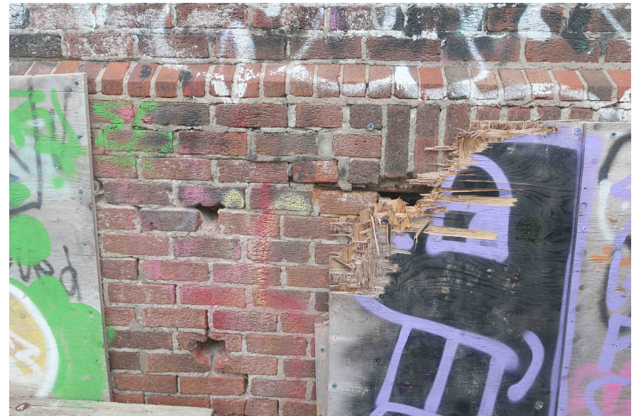
Holes in brick. This surface hoarding is damaging to the brick.
