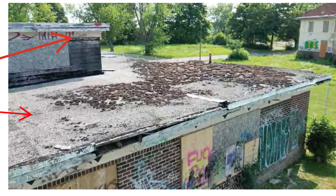
DETERIORATED ROOF SHOWING SOIL AND BIOLOGICAL GROWTH
