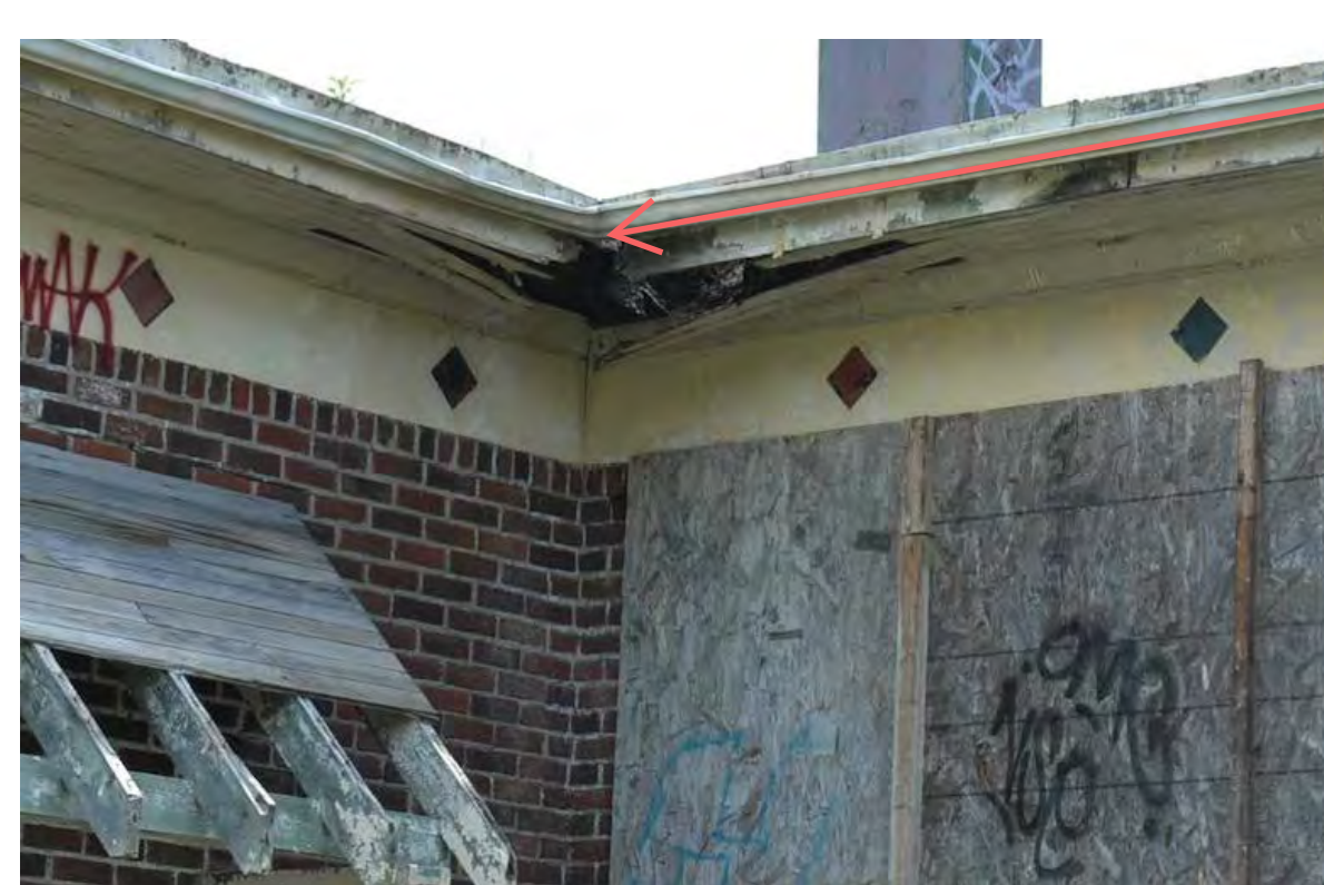
DETERIORATED FLASHING, FASCIA AND SOFFIT
