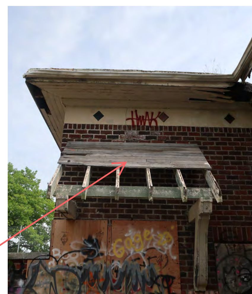
DETERIORATED CANOPY AND BRACKET
