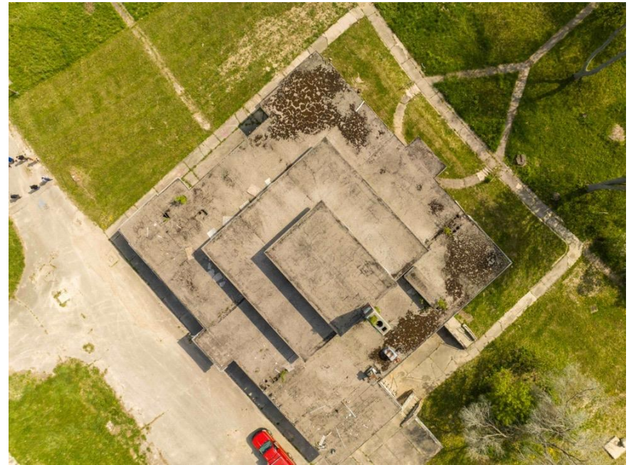
Roof Plan showing soiling at west side
