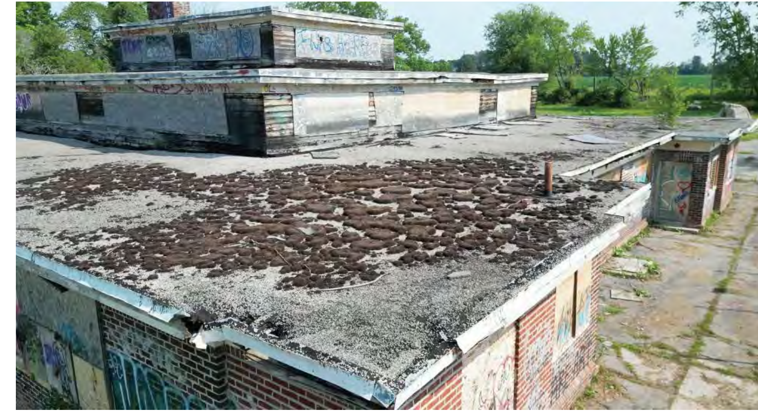
TRIPPLE HEIGHT ROOF FORM SHOWING ABSENCE OF GUTTERS DETERIORATED FLASHING AND ROOF
