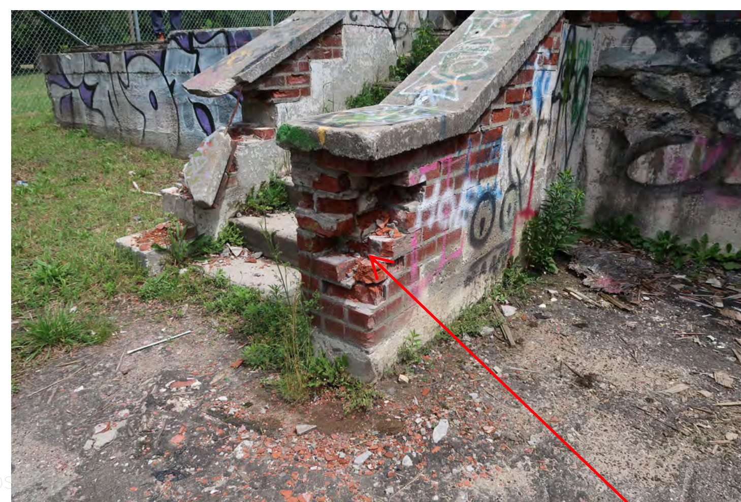
DETERIORATED EXTERIOR STAIRS
