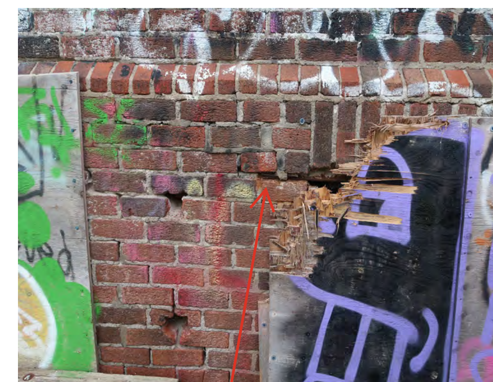
HOLES IN BRICKS
