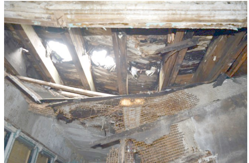
Collapsed lath and plaster ceiling including wood decking and joists.
