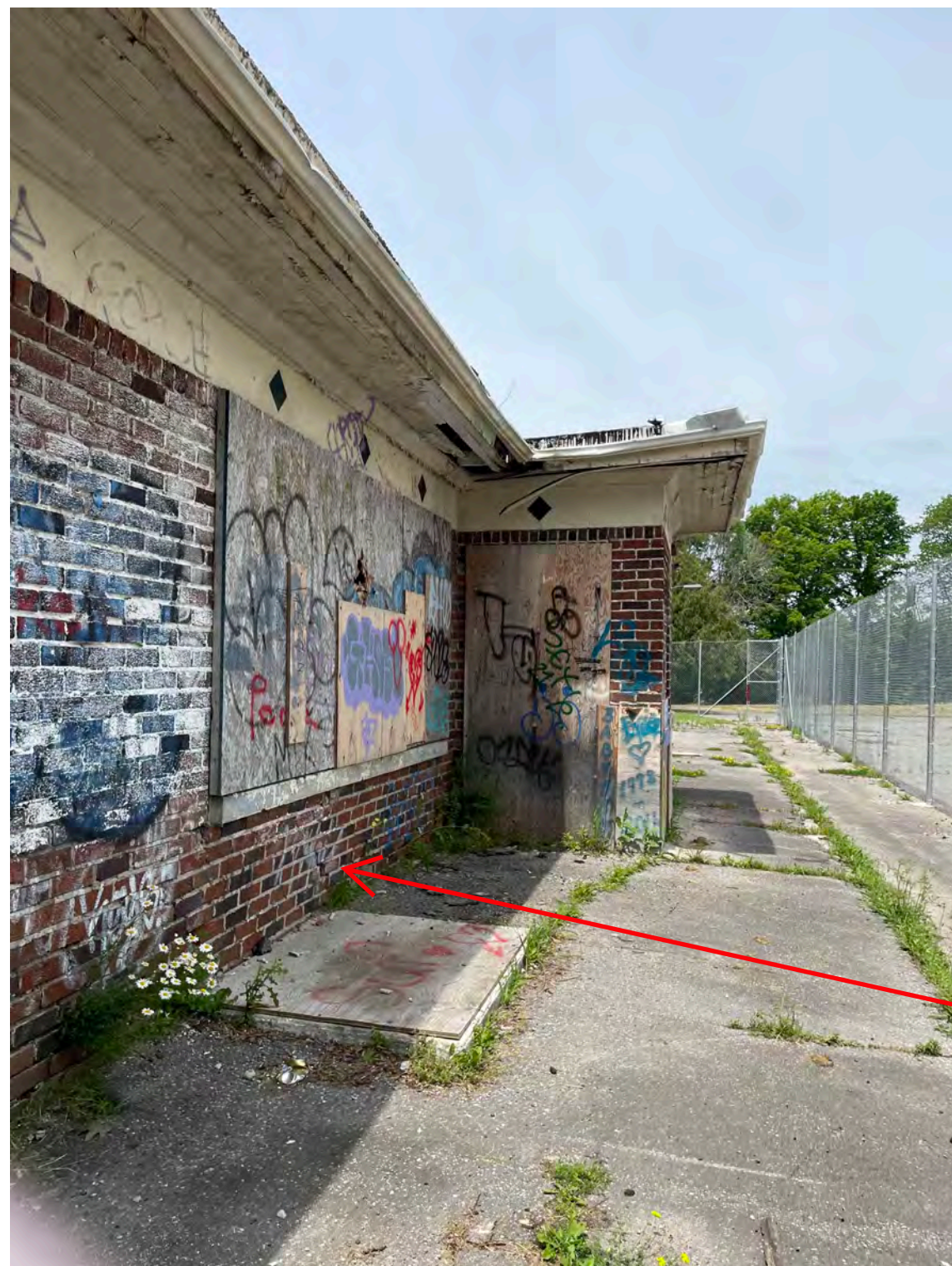
LEANING BRICK WALL
