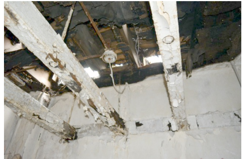
Wood ceiling joists in very poor condition where ceiling has caved in.
