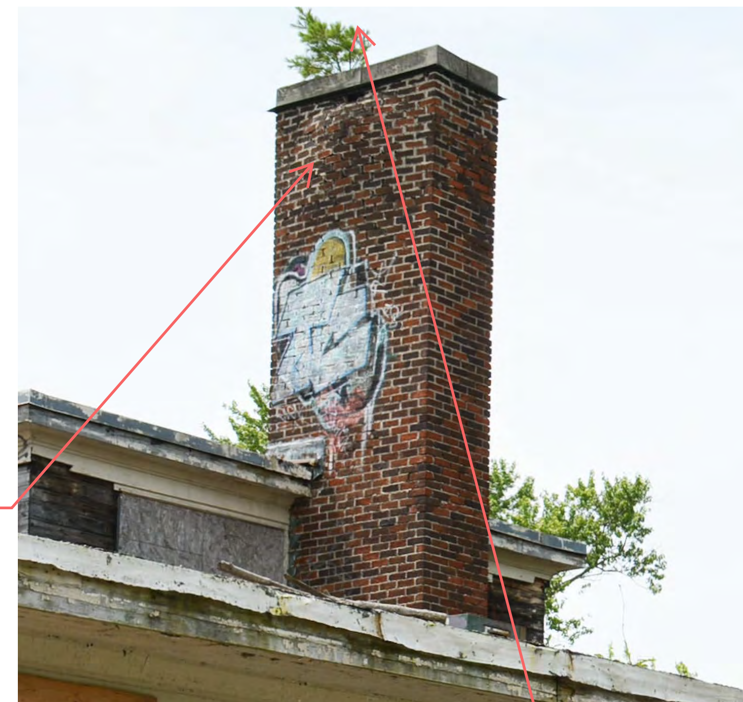
BULGING CHIMNEY AND VEGETATION GROWTH
