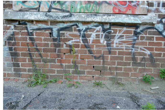
Cracks in west side wall.
