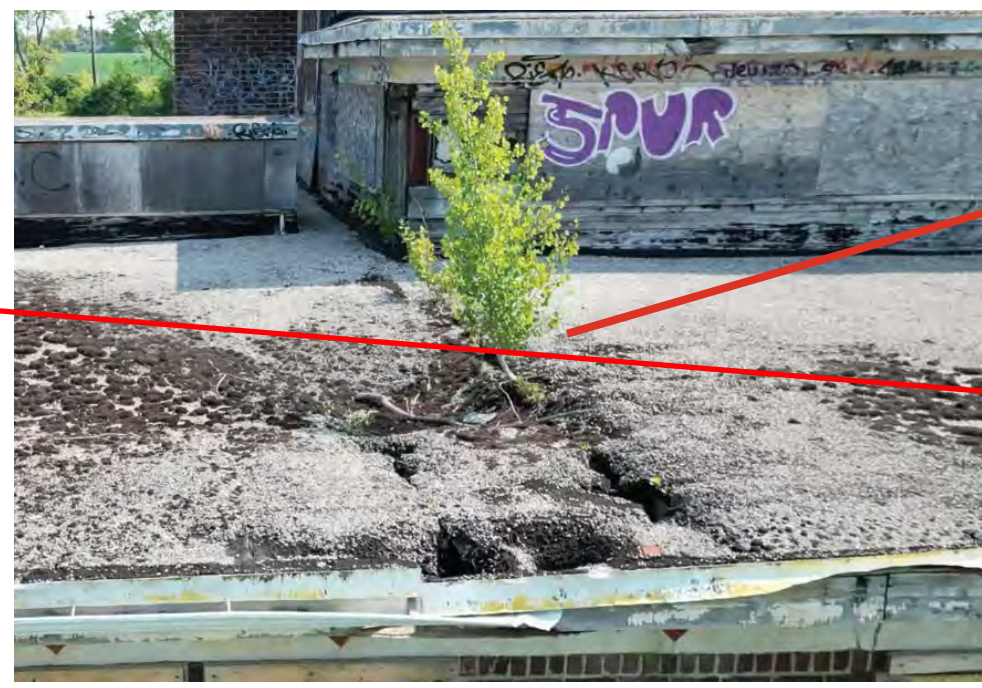
DETERIORATED ROOF CAVING IN AND BIOLOGICAL GROWTH
