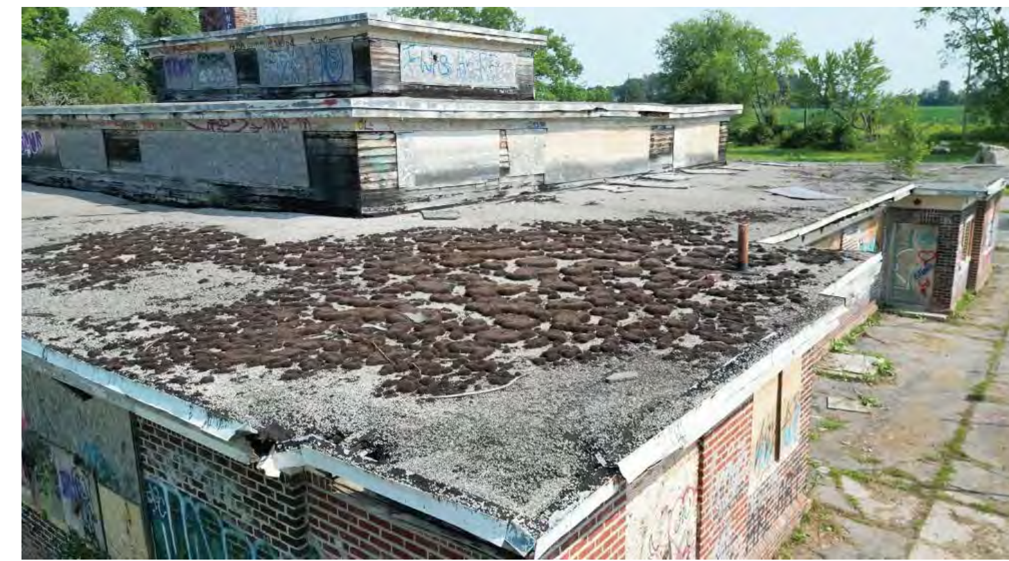
TRIPPLE HEIGHT ROOF FORM SHOWING ABSENCE OF GUTTERS DETERIORATED FLASHING AND ROOF
