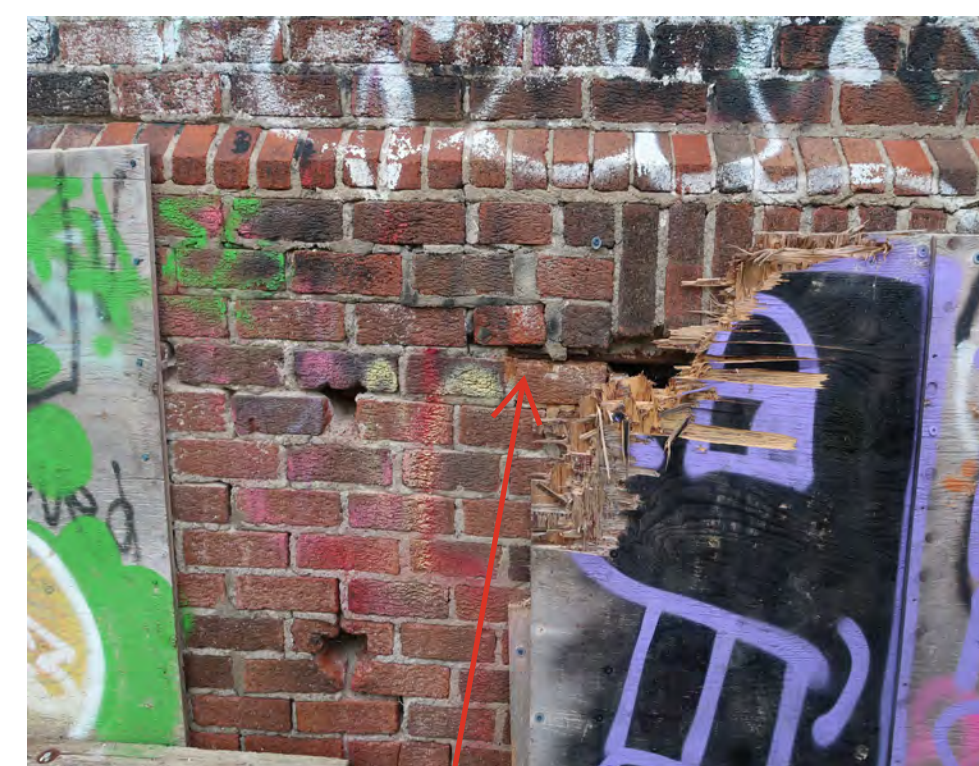
HOLES IN BRICKS
