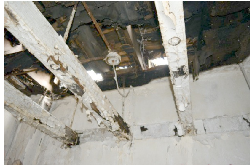
Wood ceiling joists in very poor condition where ceiling has caved in.
