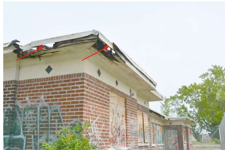
Torn flashings, missing gutter.
