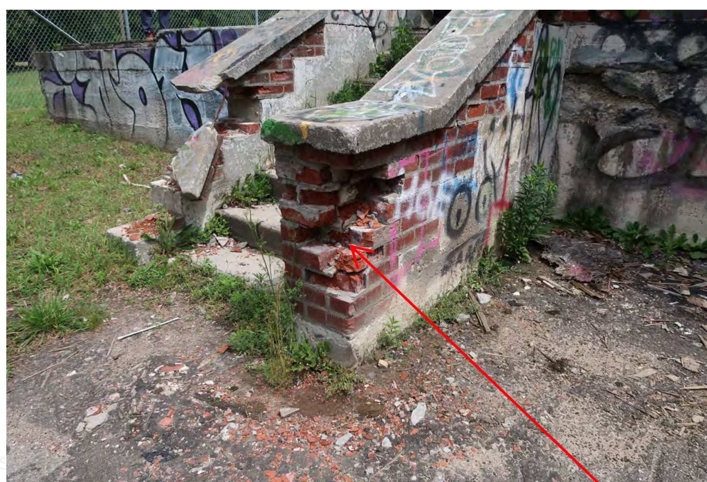
DETERIORATED EXTERIOR STAIRS
