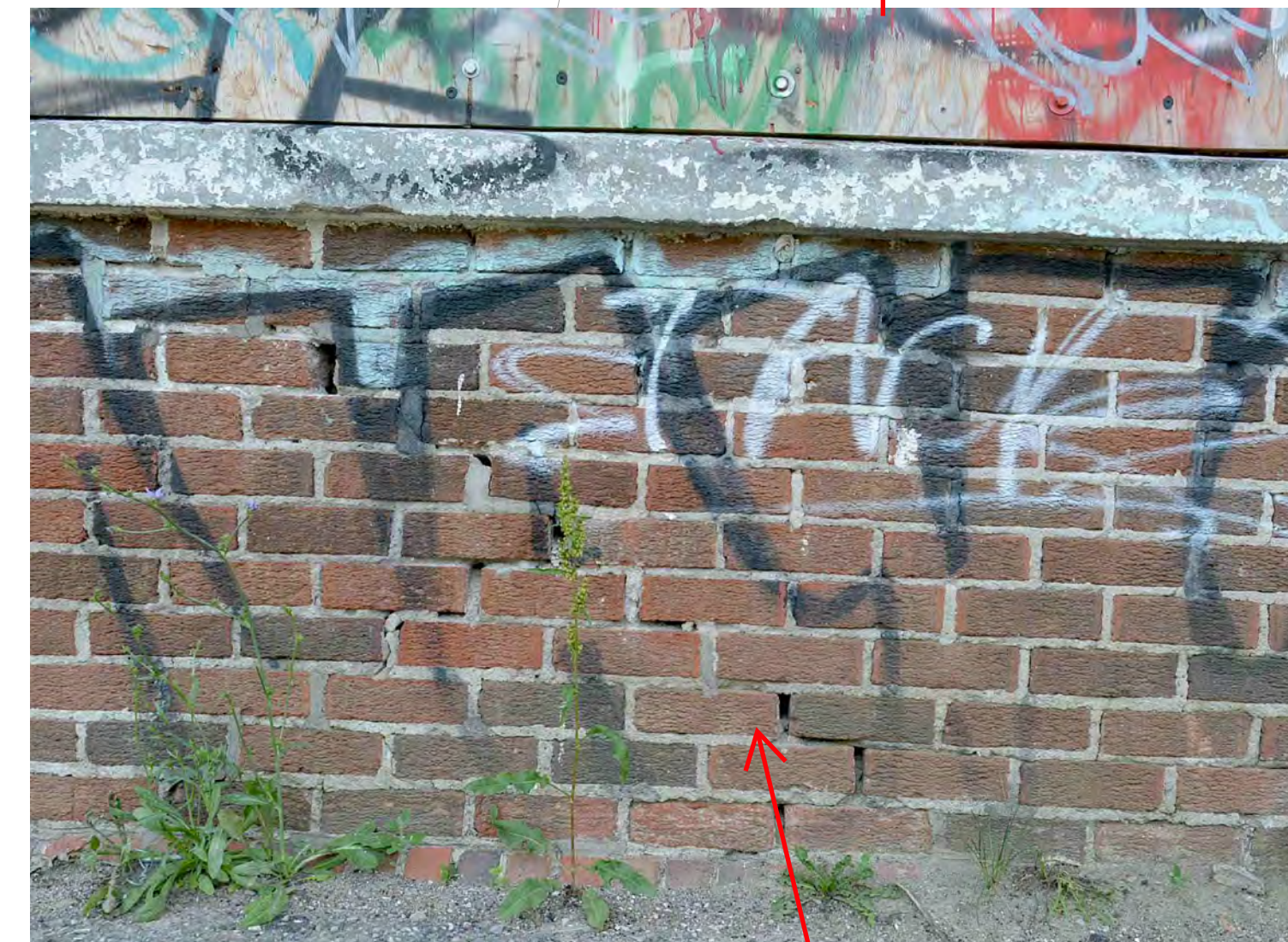
DETERIORATED MORTAR JOINTS
