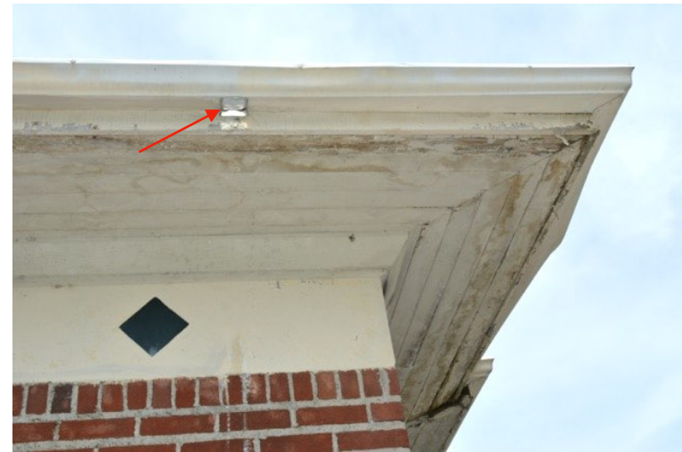
Missing rain water leaders typical.
