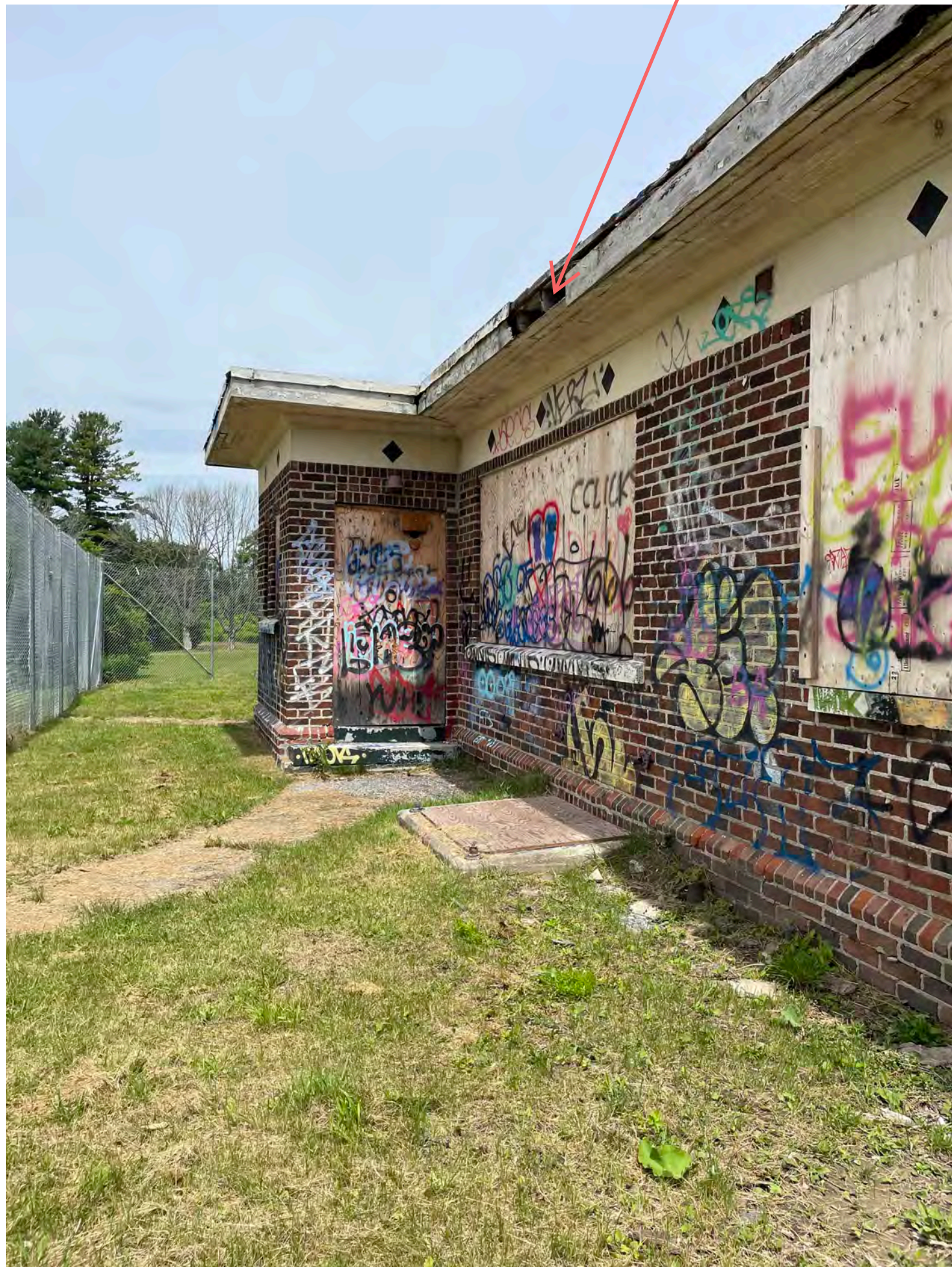
ELEVATION SHOWING VANDALISM
