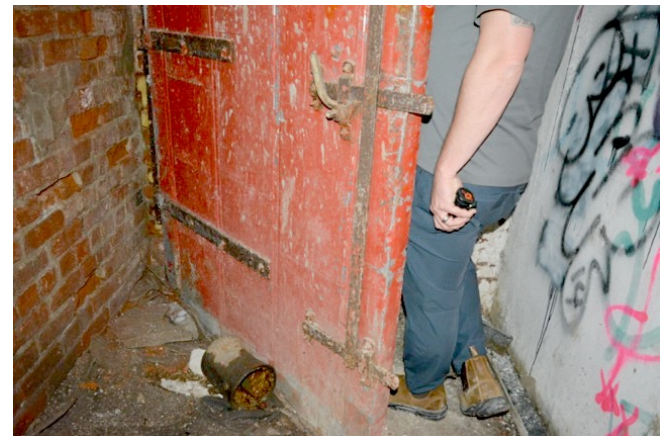
Metal door to the boiler room in the basement. A rectangular door in an arched opening.
