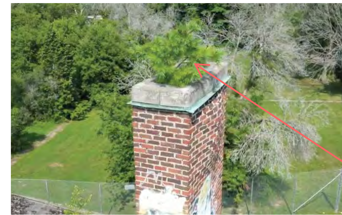
DETERIORATED CHIMNEY SHOWN SIGNS BULGING AND VEGETATION GROWTH FROM THE FLUE
