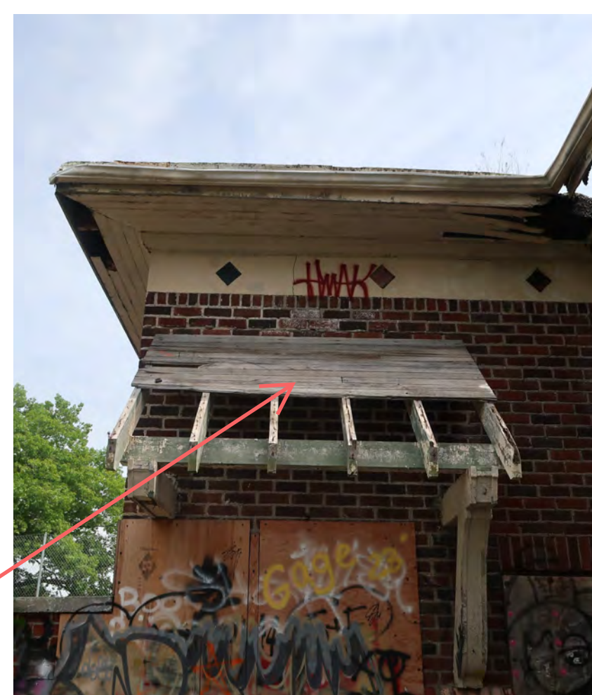
DETERIORATED CANOPY AND BRACKET
