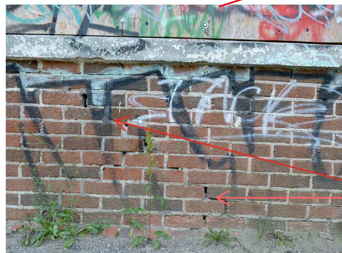
DETERIORATED MORTAR JOINTS
