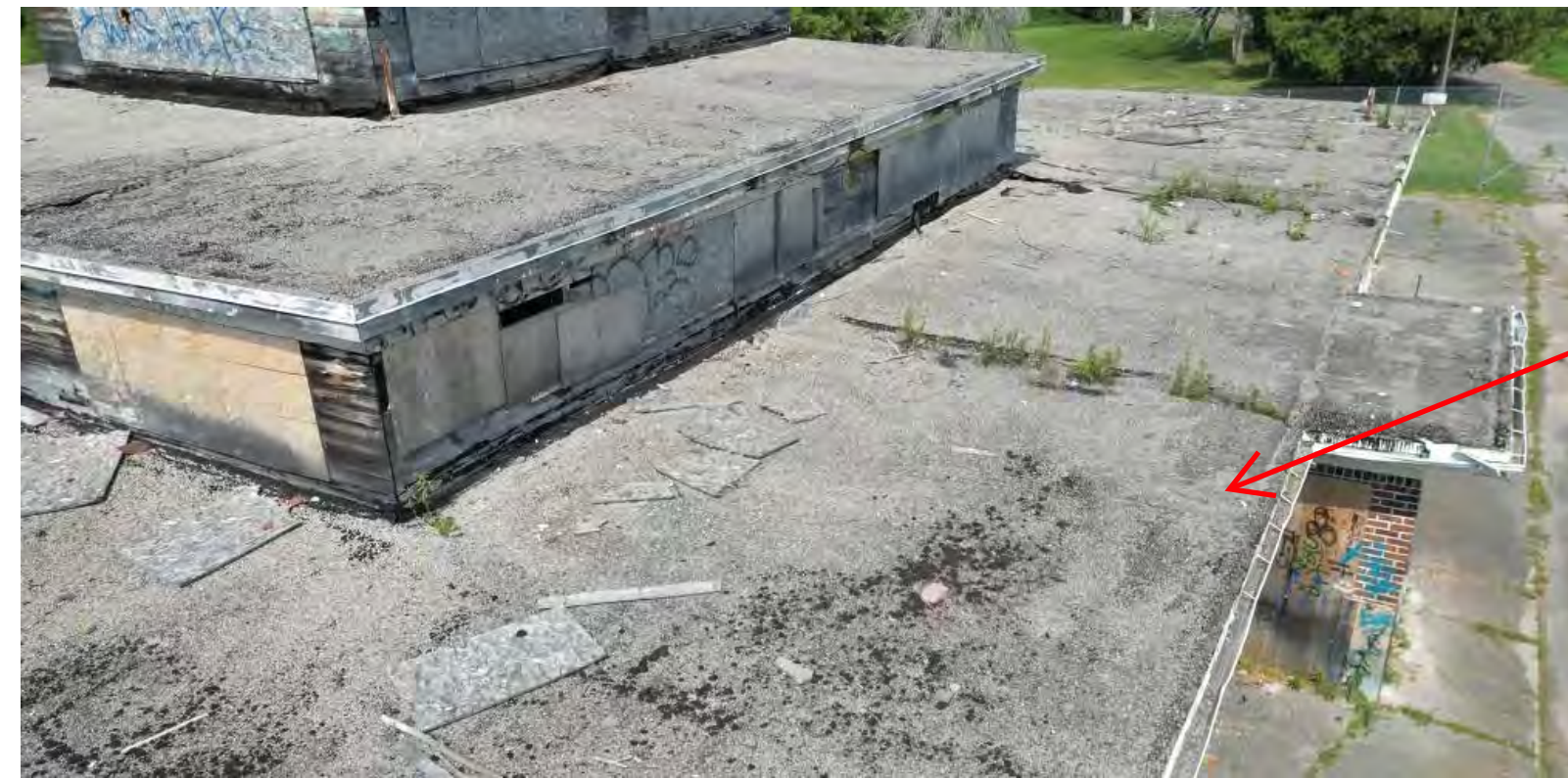
DETERIORATED ROOF AND BIOLOGICAL GROWTH
