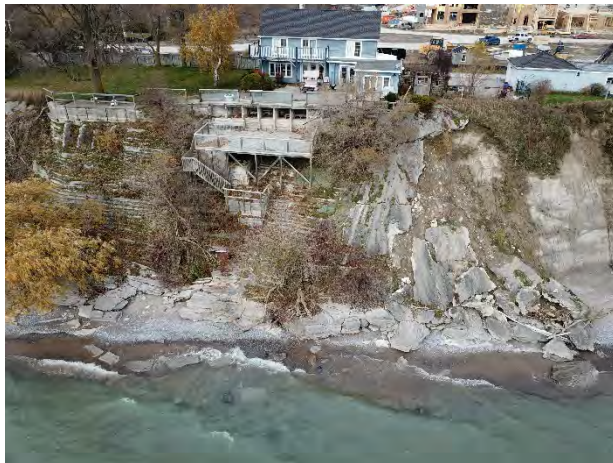
Eroding Bluffs and Failed Shore Protection East of Port Darlington
