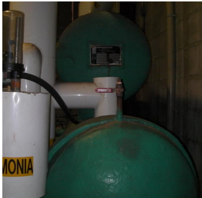
Figure 1: Chiller barrel and vessel.
