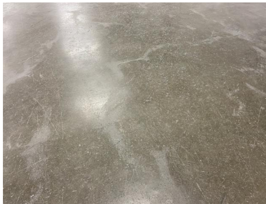
Figure 9: Scuff marks and scrapes throughout the ice rink floor
