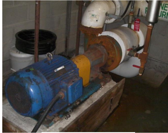
Figure 5: Cold Brine Pump
