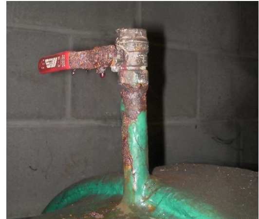
Figure 2: Signs of rusting on the chiller.
