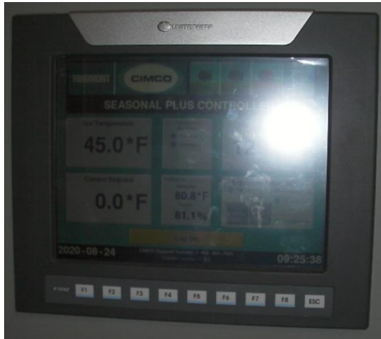
Figure 7: Primary Control Panel
