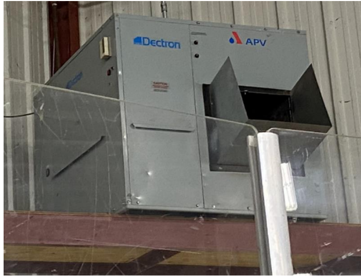
Figure 15: Mechanical dehumidifier in rink zone
