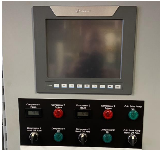
Figure 7: Primary Control Panel
