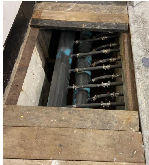
Figure 11: Clamped ice rink header with missing insulation in trench
