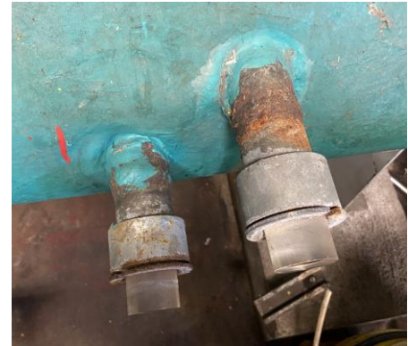
Figure 2: Signs of rusting on the chiller sight glass ports.
