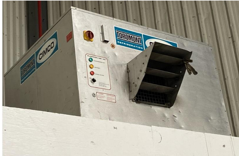
Figure 15: Mechanical dehumidifier in rink zone
