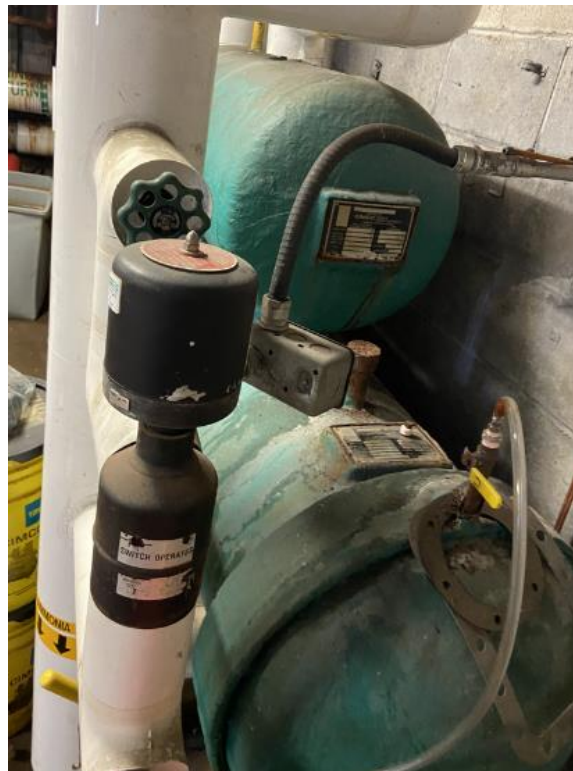
Figure 1: Chiller barrel and vessel.
