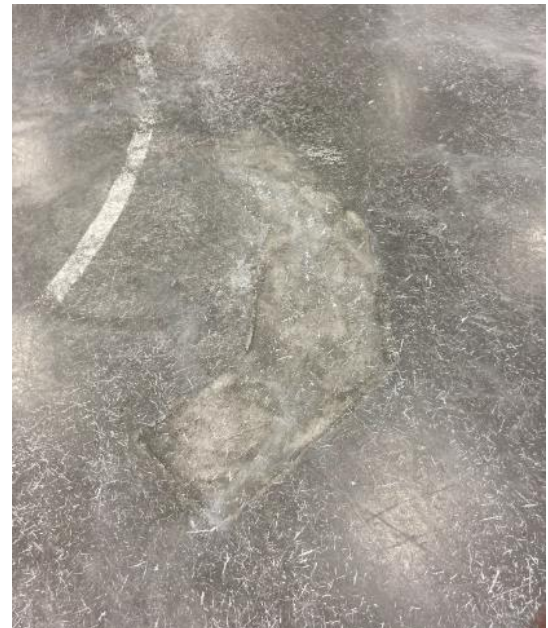
Figure 10: Scrapes and divots noted over ice rink floor surface
