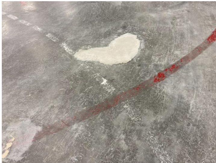
Figure 9: Ice rink floor showing serious signs of wear
