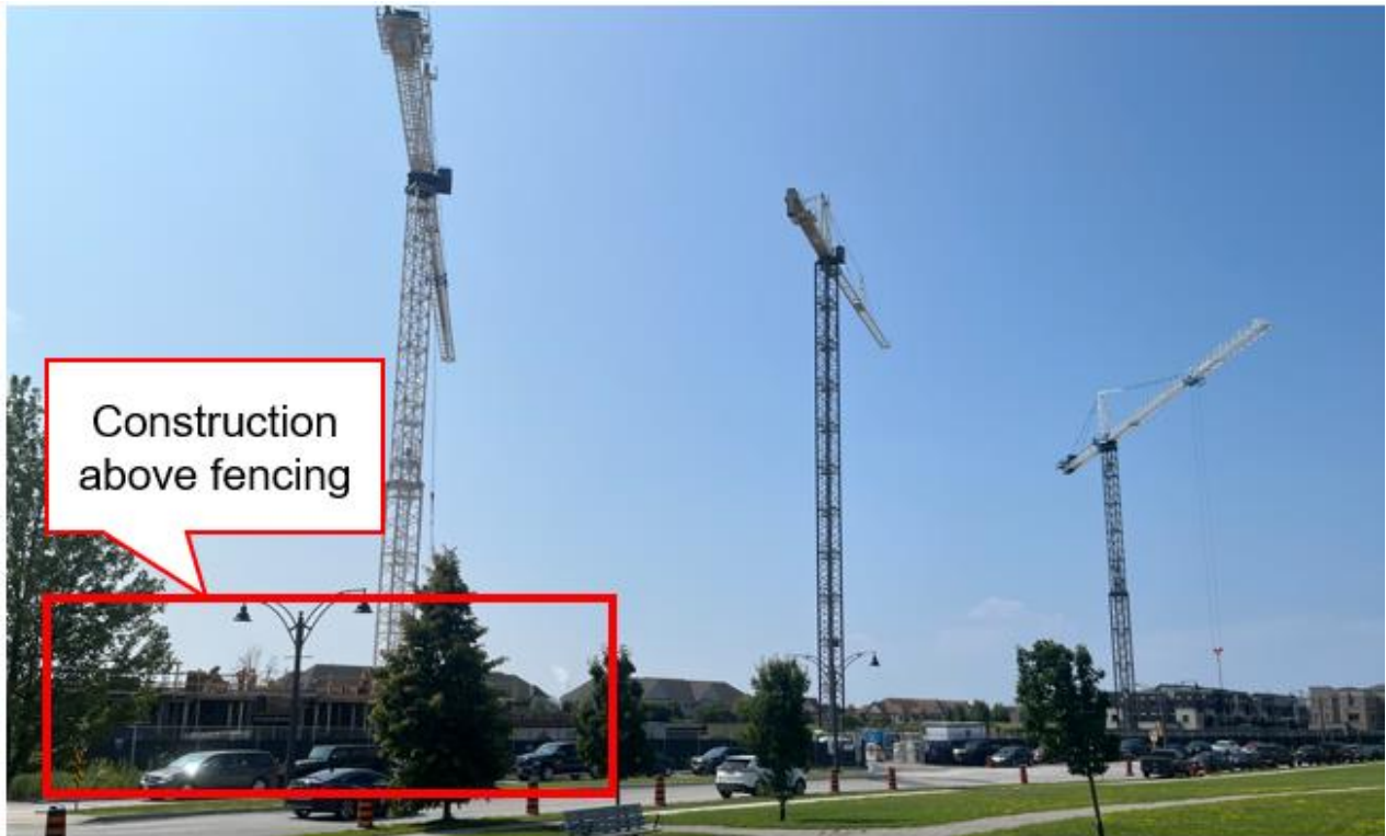
Figure 3: Image from July 2023 of 51 and 55 Clarington Boulevard (Construction above ground and active construction site)
