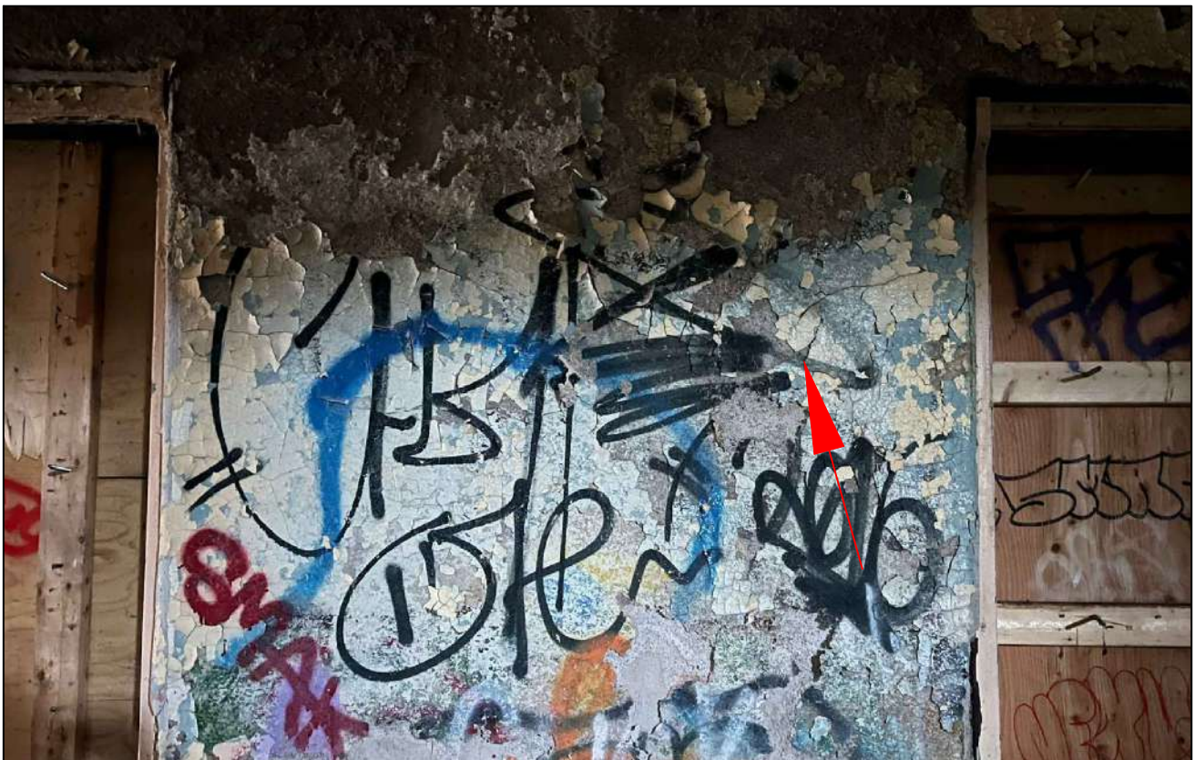
Photograph 18 Lead Containing paint on Interior South Wall
