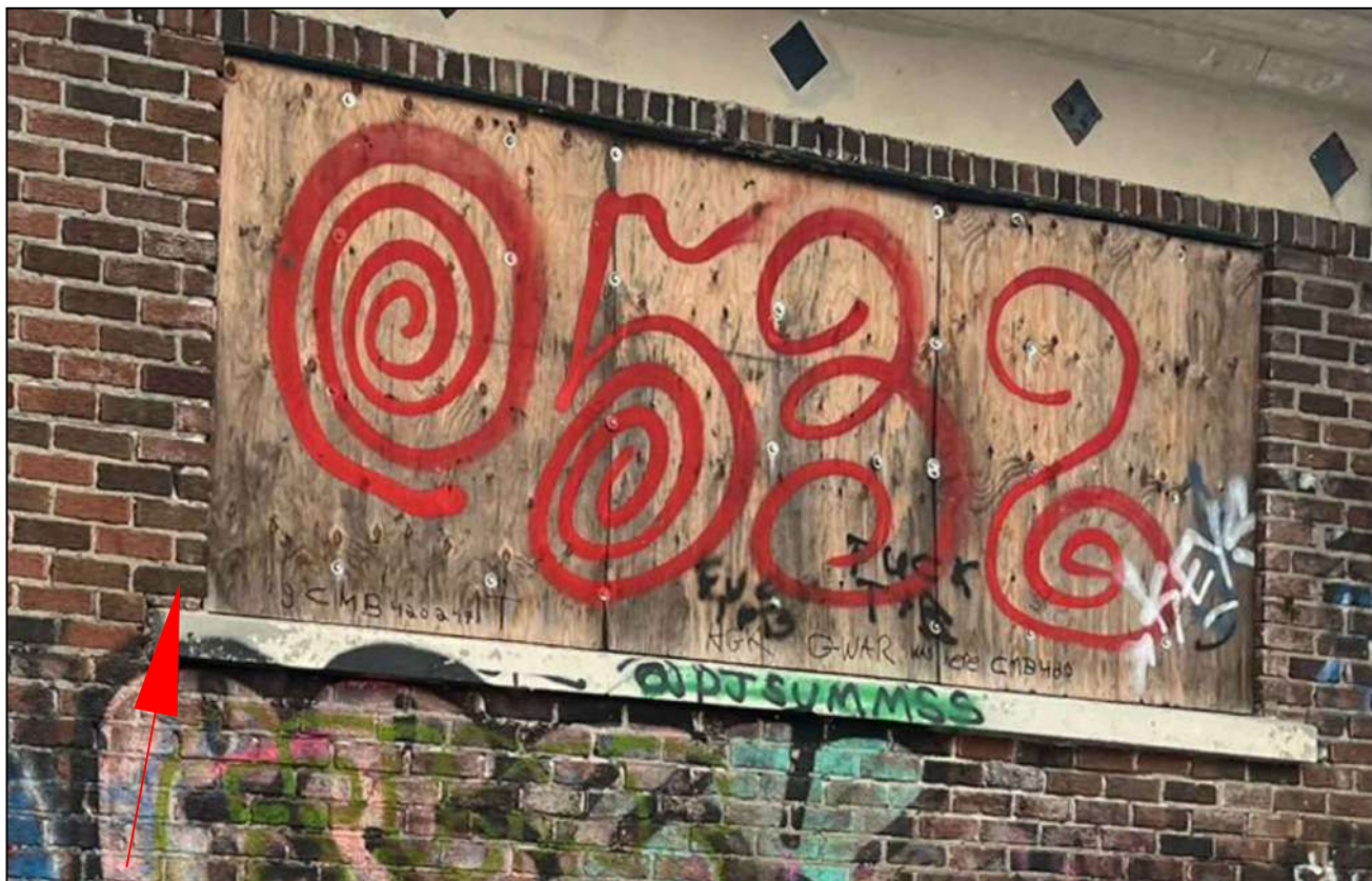
Photograph 11 Asbestos Containing on Window Caulking on Exterior East Wall
