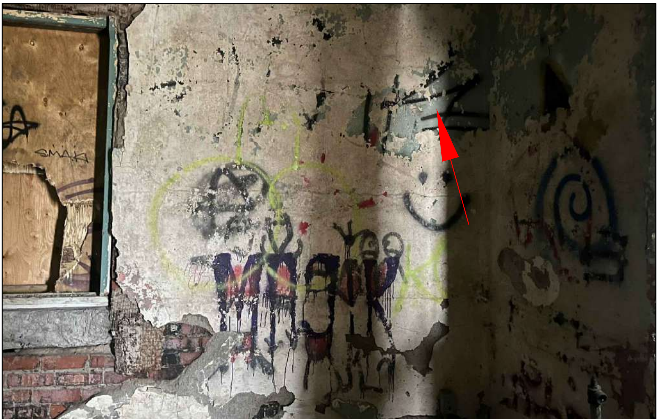
Photograph 16 Lead Containing paint on South East Interior Wall
