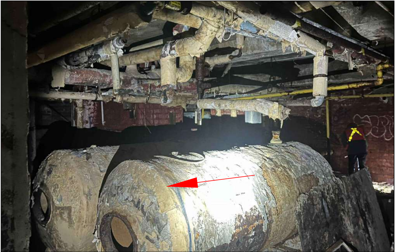
Photograph 1 Asbestos Containing Boiler Insulation
