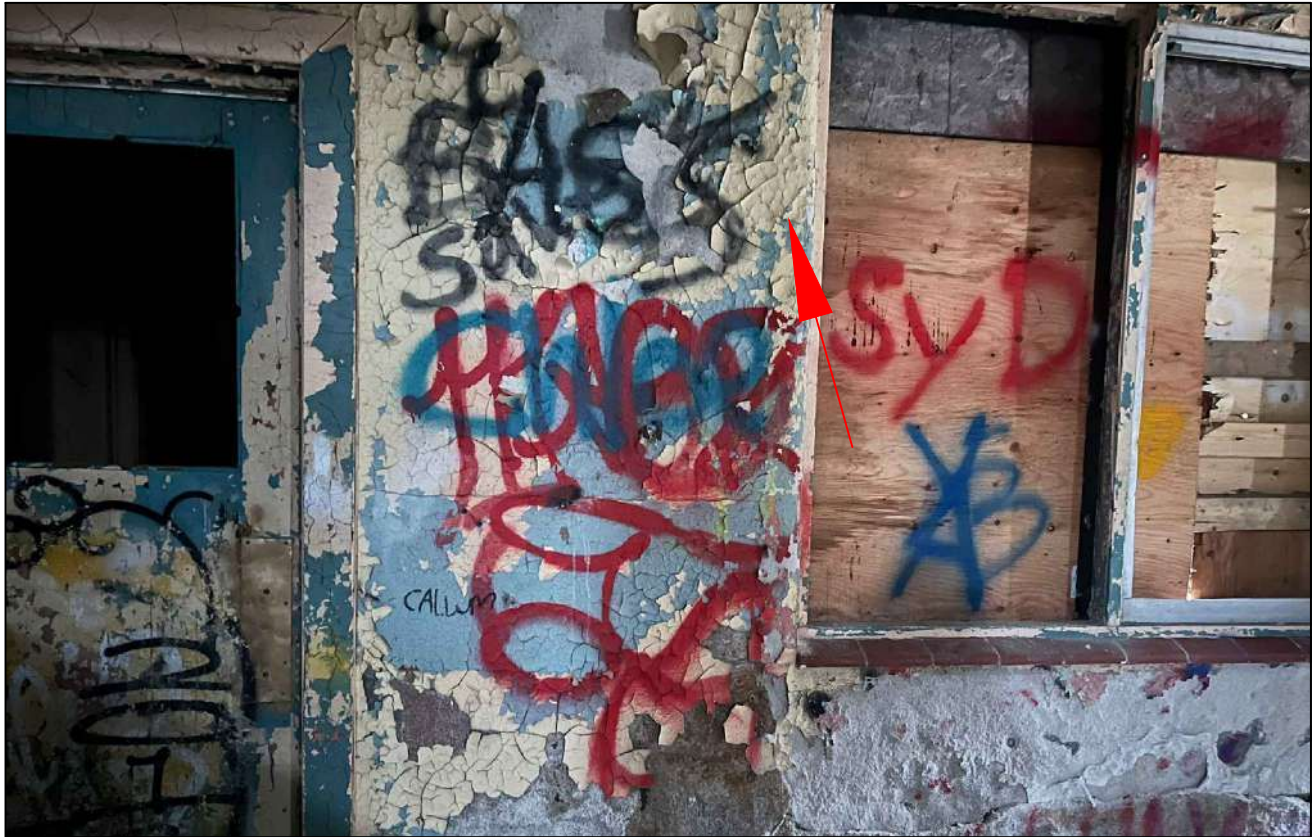
Photograph 19 Lead Containing paint on Interior West Wall
