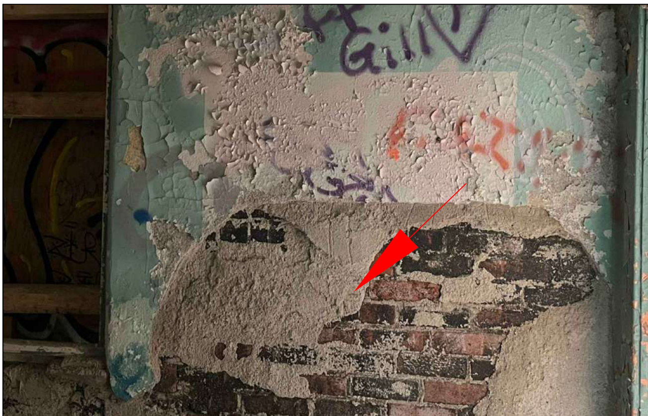
Photograph 8 Asbestos Containing Flat Plaster on Interior North wall at Entrance
