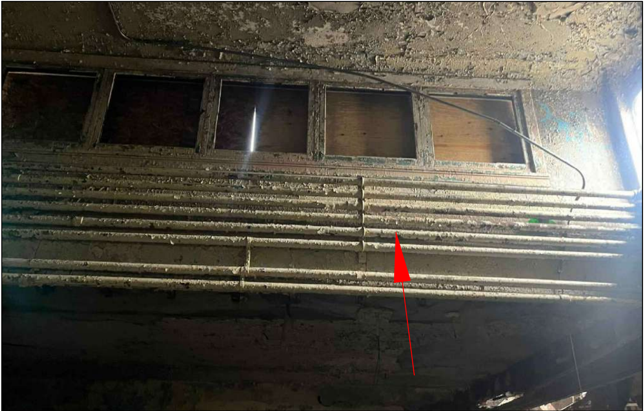
Photograph 15 Peeling Lead Containing paint on Hot Water Lines
