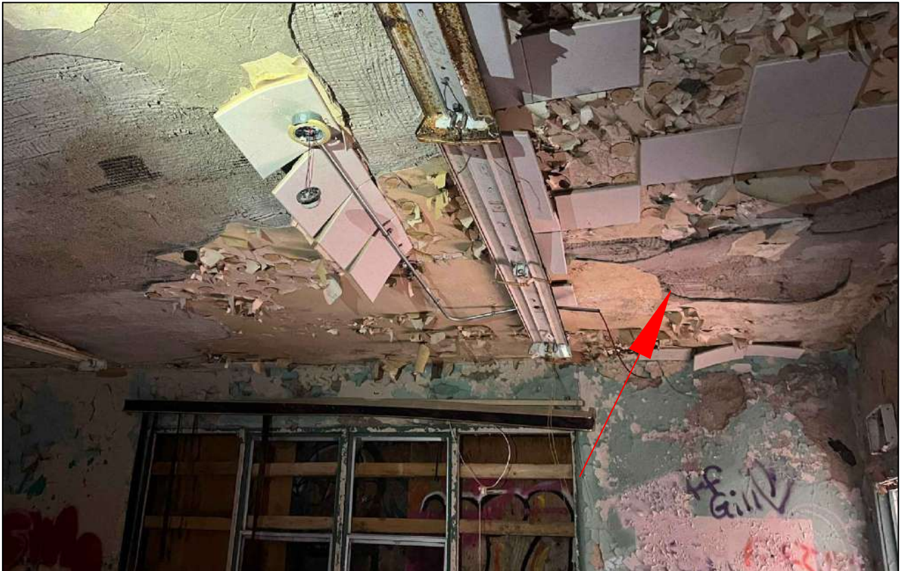
Photograph 10 Asbestos Containing Lower Ceiling Plaster on Interior North West wall
