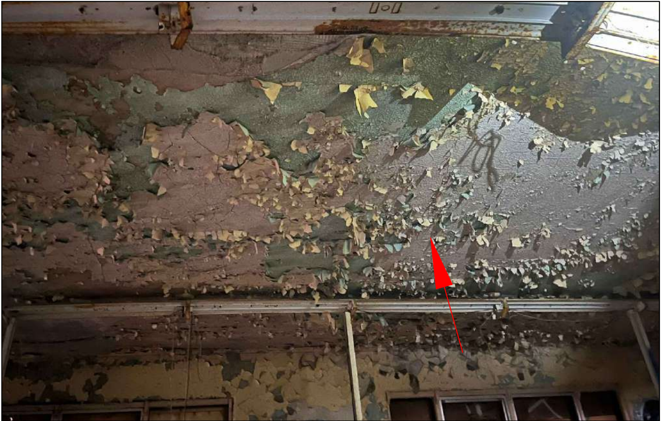
Photograph 17 Lead Containing paint on Interior South Lower Ceiling
