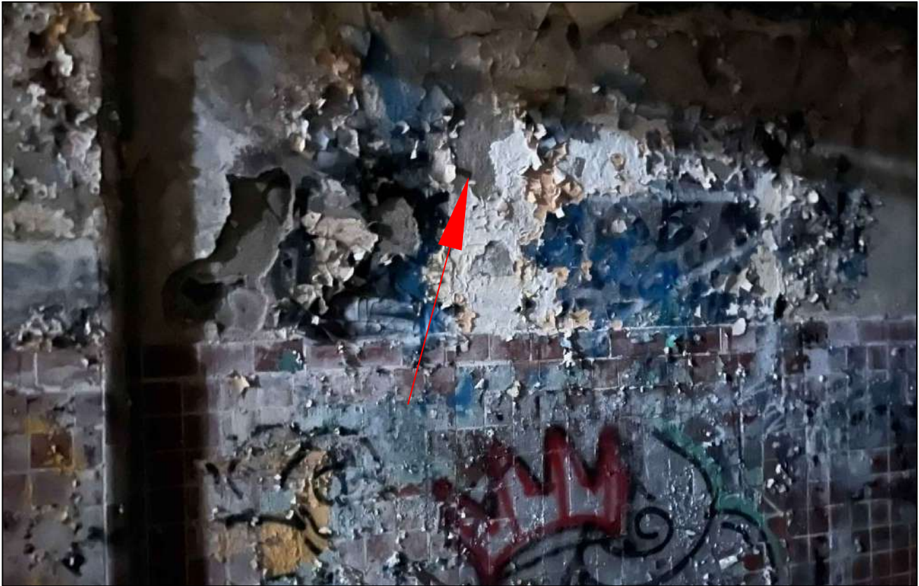
Photograph 9 Asbestos Containing Flat Plaster on Kitchen Wall
