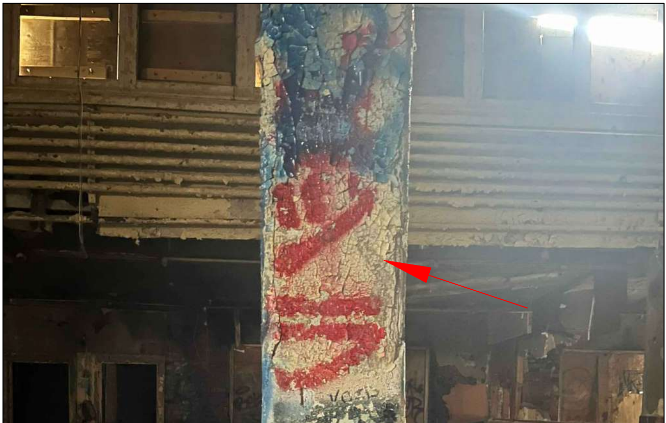
Photograph 20 Lead Containing paint on South East Column
