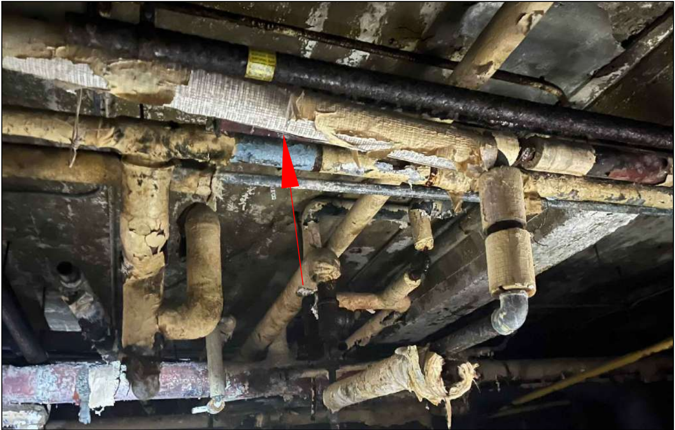
Photograph 3 Air-Cell and Parging Cement Insulation in Boiler Room
