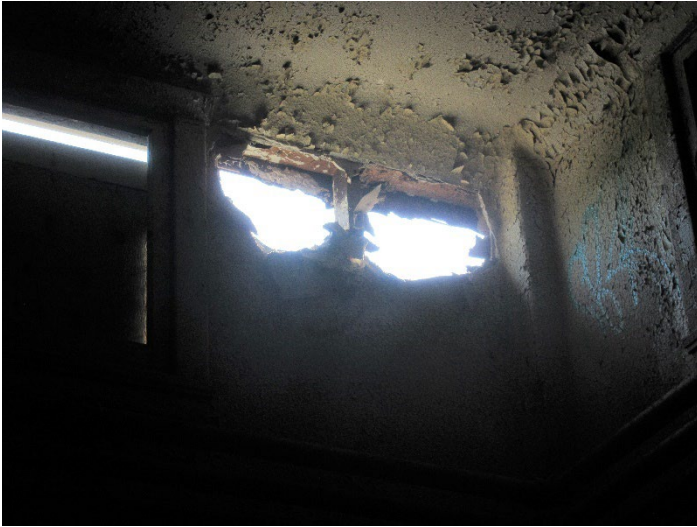
Photo 009 – Failure of Exterior Cladding
