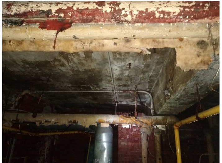
Photo 012 – Moisture Infiltration of Suspended Slab
