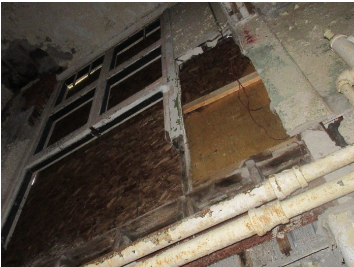
Photo 011 – Boarded Windows of Clerestory
