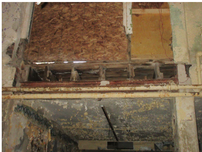
Photo 005 – Exposed Transfer Beam with Water Damage Visible
