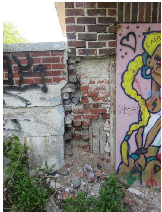
Photo 016 – External Brick Masonry Wall Damage (1/3)
