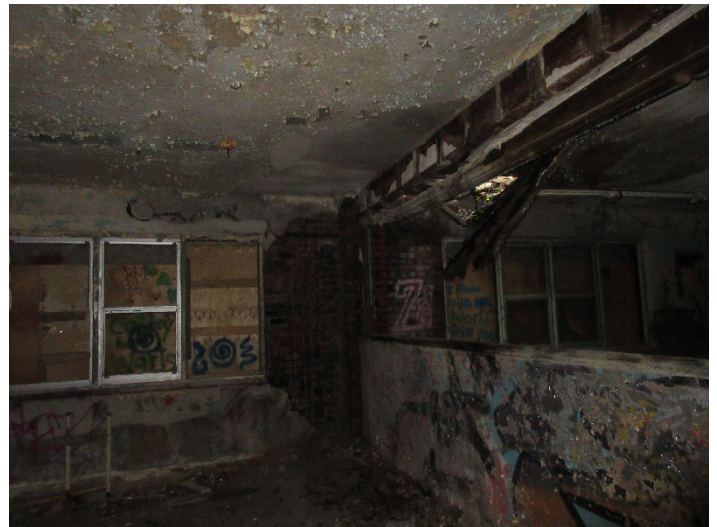
Photo 004 – Excessive Deterioration and Local Failure of Rafters (2/2)
