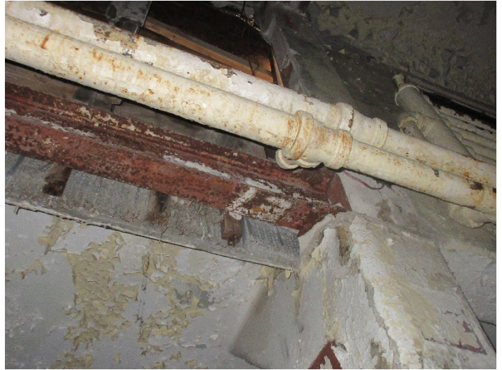
Photo 010 – Corrosion of Exposed Transfer Beam Supporting Clerestory
