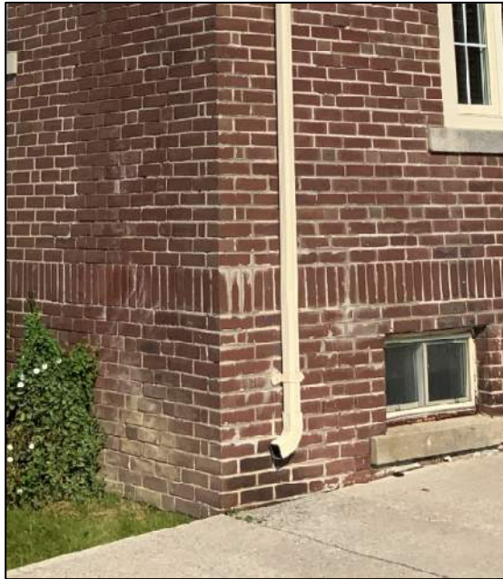
Photograph 4: Poorly executed masonry repairs (typical)
