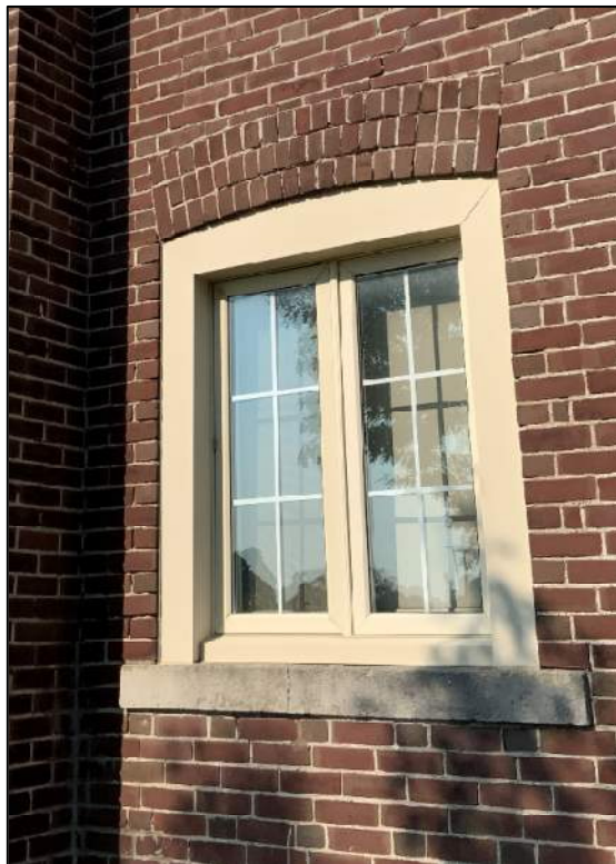
Photograph 5: Lost mortar in head joints of arch (typical)
