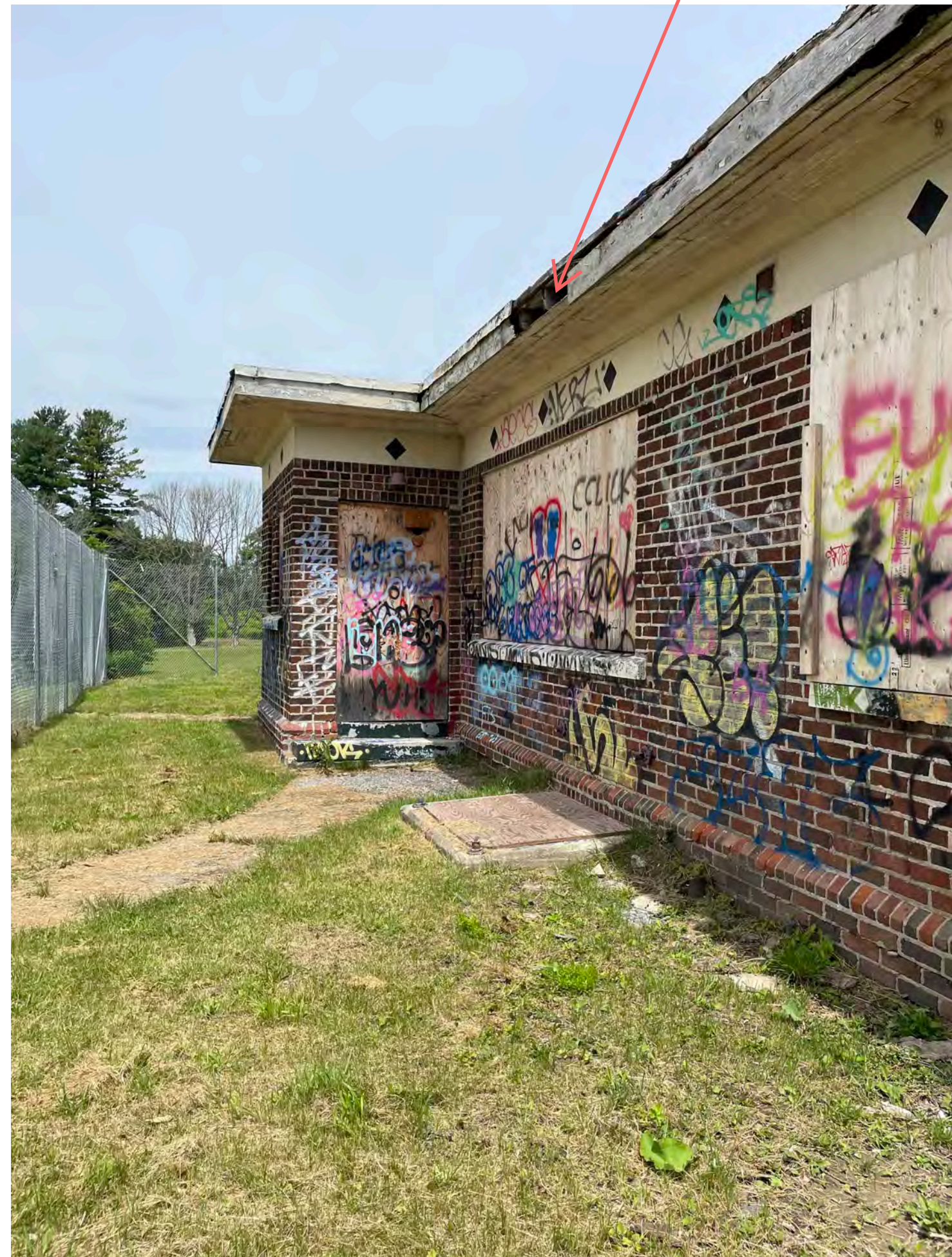
ELEVATION SHOWING VANDALISM
