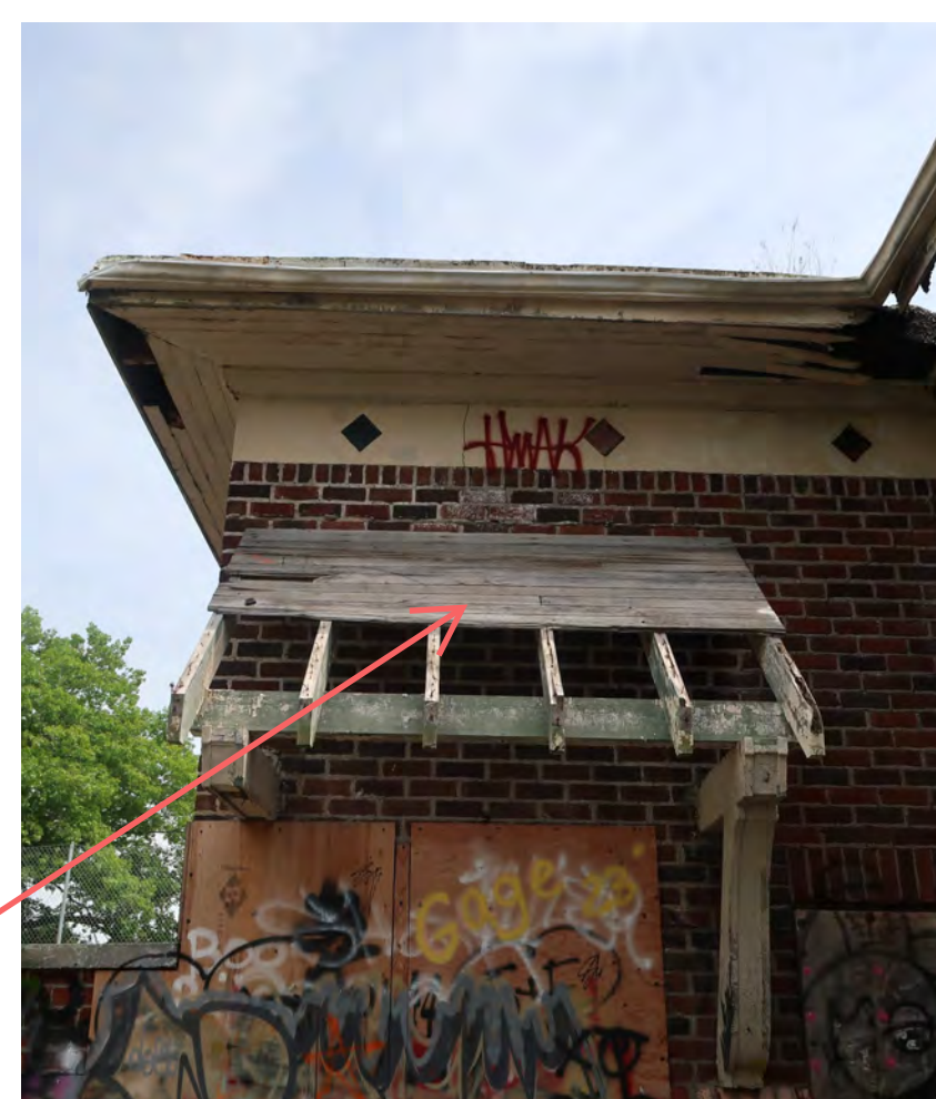
DETERIORATED CANOPY AND BRACKET
