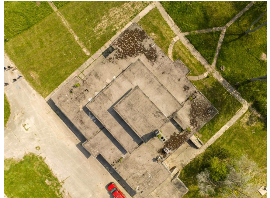
Roof Plan showing soiling at west side
