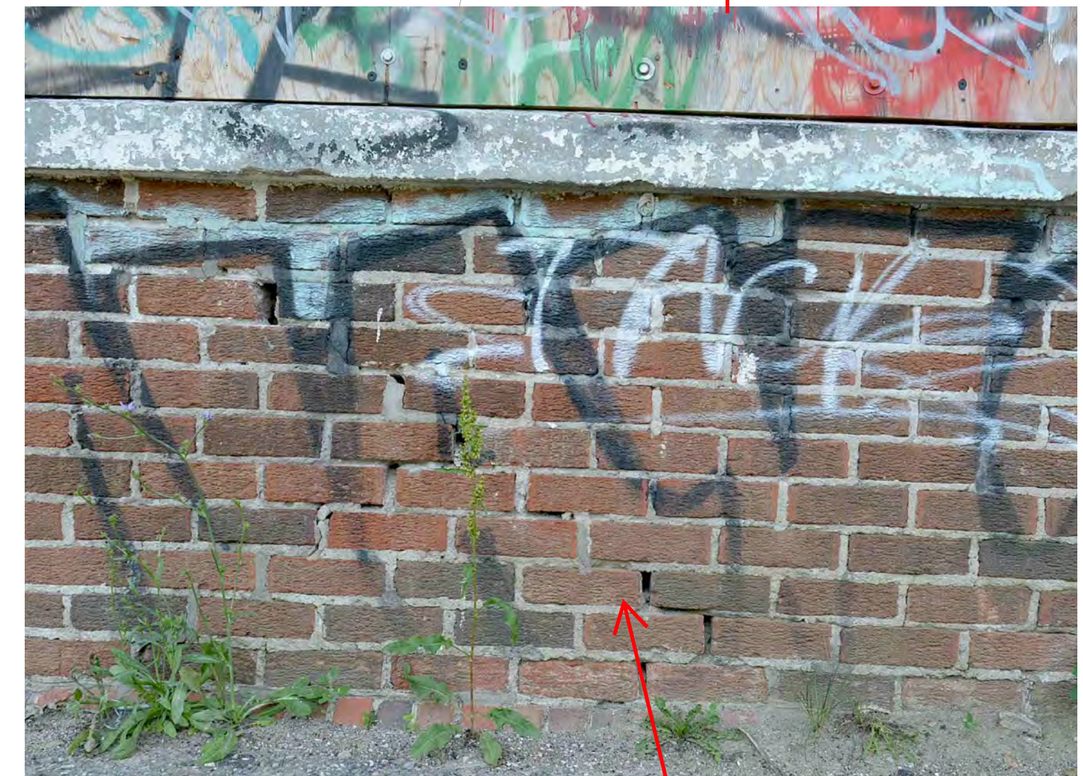
DETERIORATED MORTAR JOINTS
