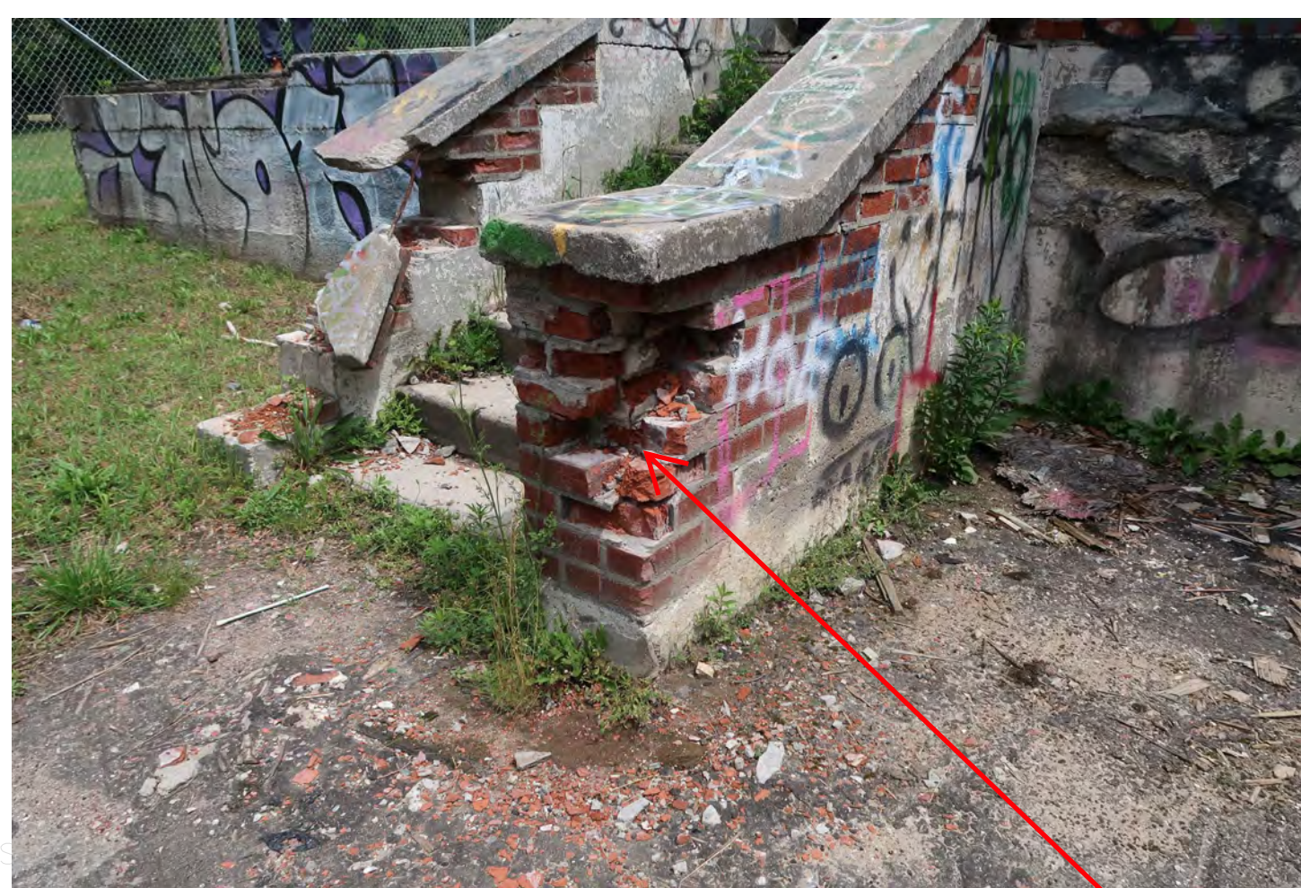
DETERIORATED EXTERIOR STAIRS
