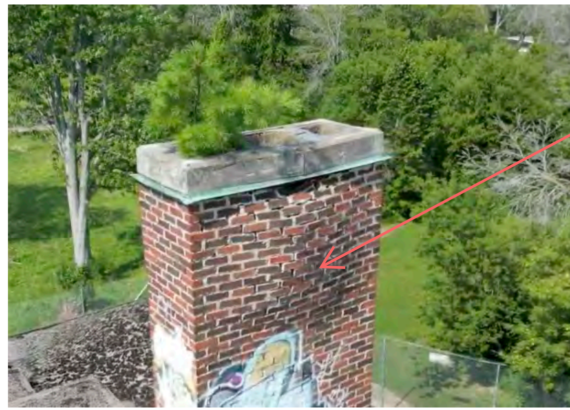
DETERIORATED CHIMNE SHOWN SIGNS BULGING AND VEGETATION GROWTH FROM THE FLUE
