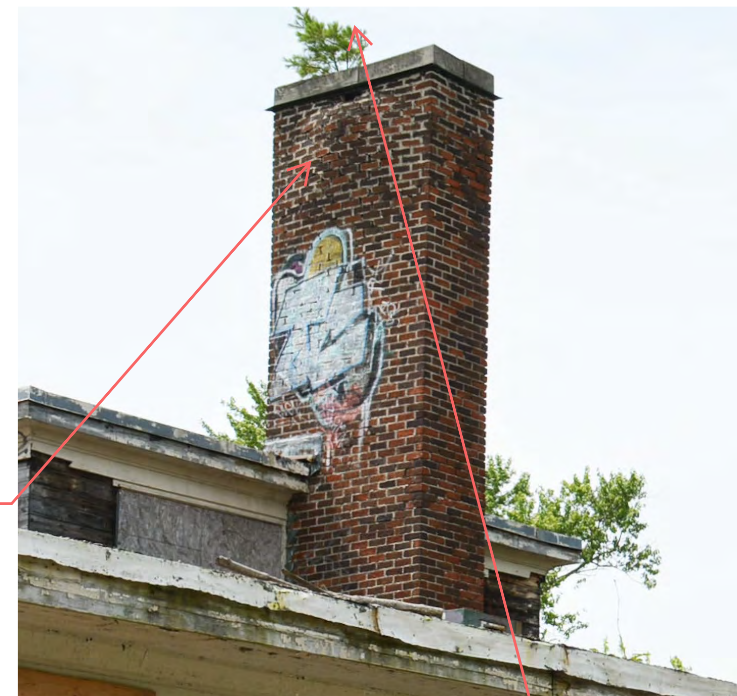
BULGING CHIMNEY AND VEGETATION GROWTH
