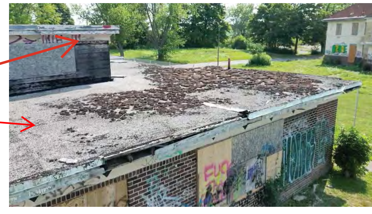
DETERIORATED ROOF SHOWING SOIL AND BIOLOGICAL GROWTH
