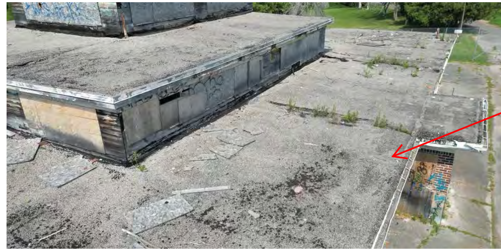
DETERIORATED ROOF AND BIOLOGICAL GROWTH
