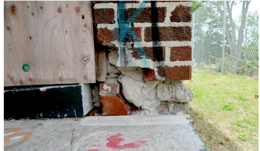
Broken bricks around doorway sills in a few locations requiring reconstruction.
