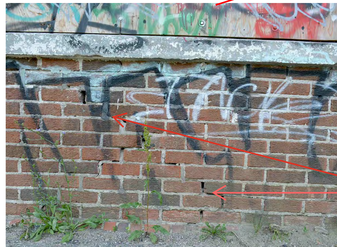
DETERIORATED MORTAR JOINTS
