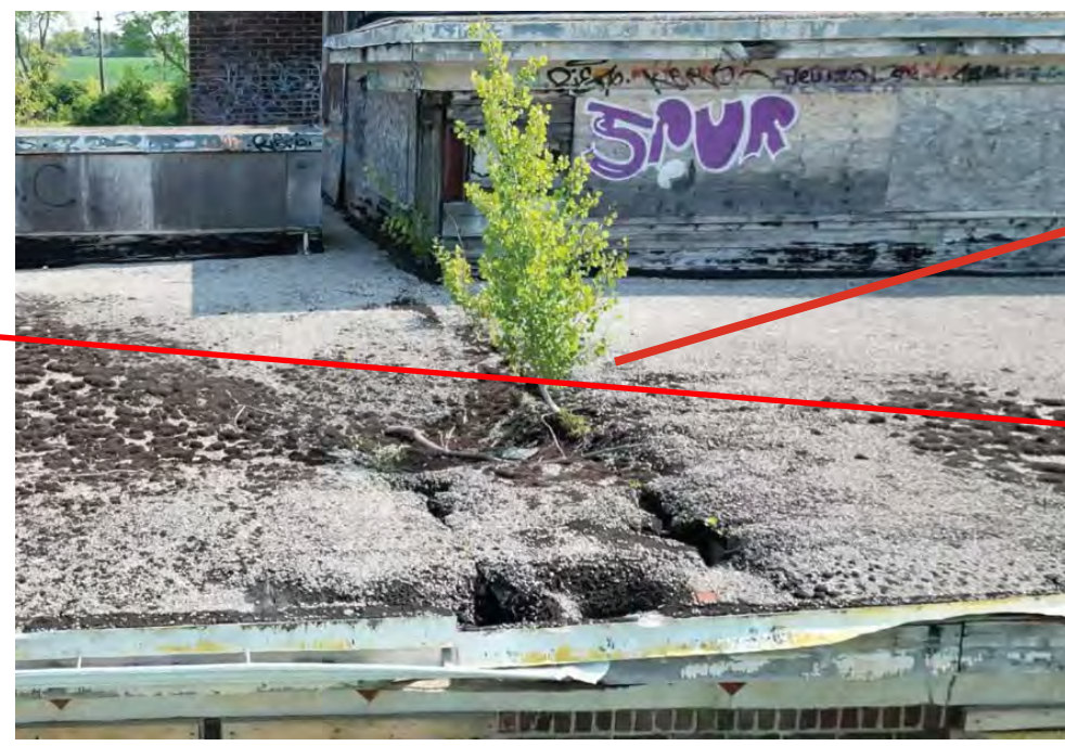
DETERIORATED ROOF CAVING IN AND BIOLOGICAL GROWTH
