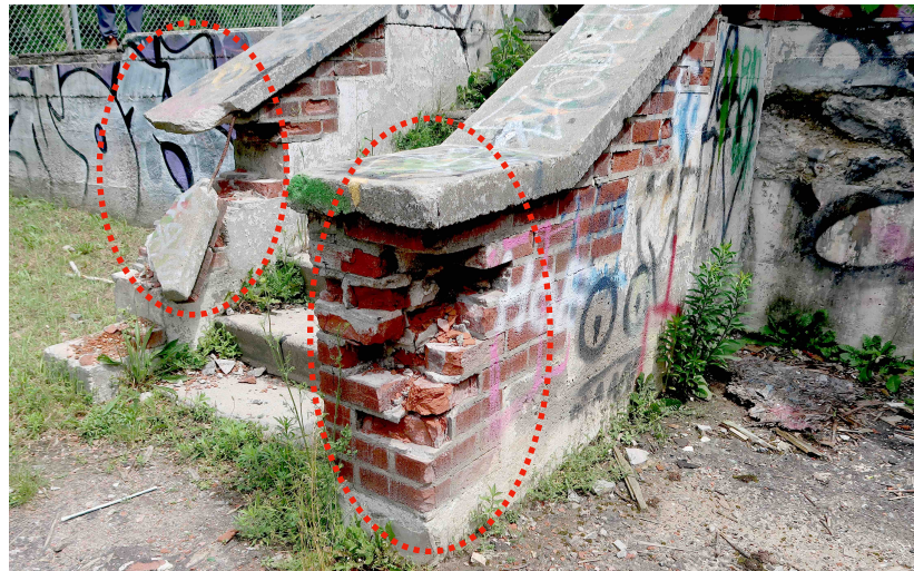
Steps on north side extensively deteriorated and may have been subjected to vandalism
