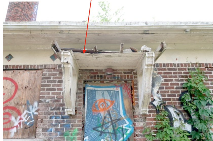
Remains of Canopy roof facing north.
