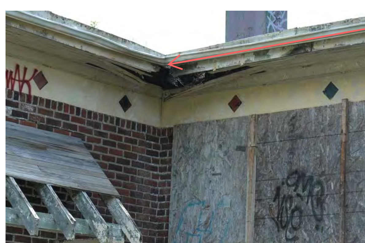
DETERIORATED FLASHING, FACSIA AND SOFFIT
