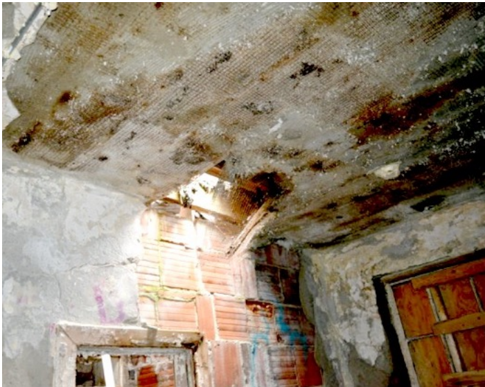
Mold apparent in lath and concrete ceilings.
