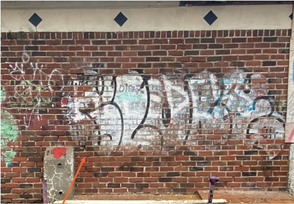
Deteriorated mortar joints
