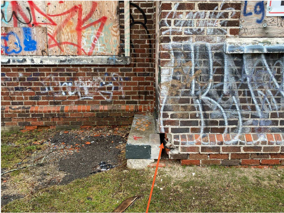
Deteriorated mortar and collapsed brick
